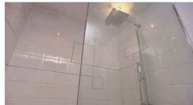
Detail of graphic detail on walls and designer shower head
